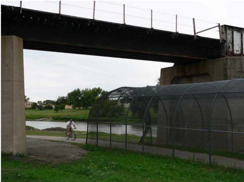
Figure 12: Integrated chain-link cover and fencing protects trail users along East Grand Forks National Recreation Trail in Minnesota; photo courtesy Stuart Macdonald
